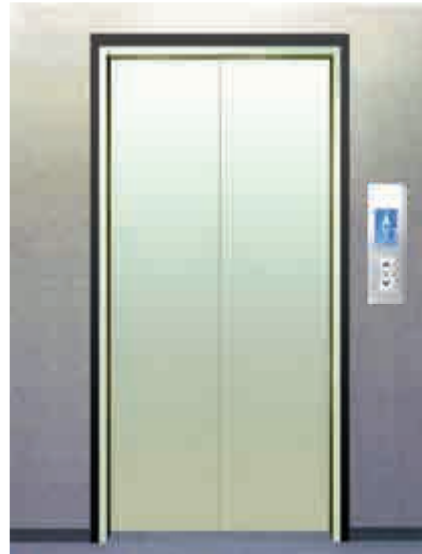
Porta de Andar: apple green painted steel plate (standard for the typical floor)
